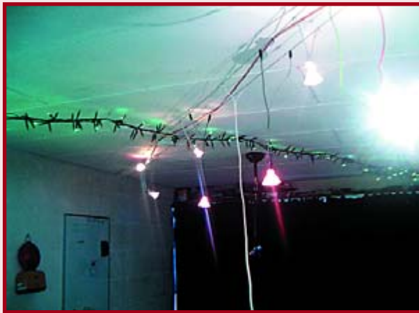
9. The power-on surge with so many lights can be quite high indeed.
