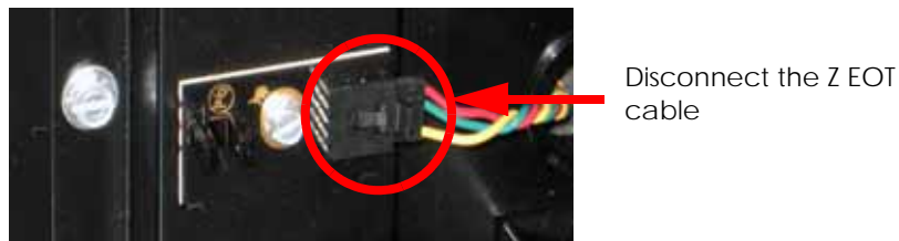
Figure 4-240: Z EOT sensor cable location
