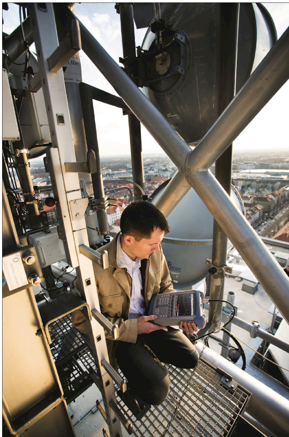
Figure 2. Cost efficient mobile T&M equipment is used to install a base station.
