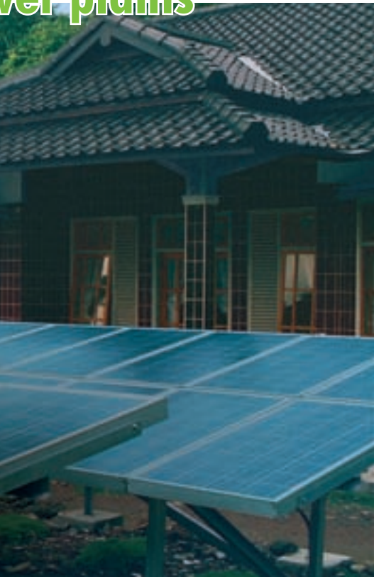
Standalone solar power installations play a vital role in regions lacking significant electrical infrastructure. This is a 4.2 kW setup in Indonesia (photo: Schott Solar GmbH).
