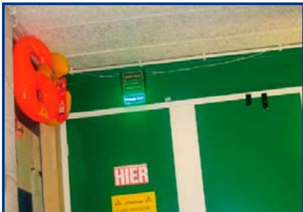
This is the final result. The electronics have been mounted inside the toilet to keep them out of sight.
