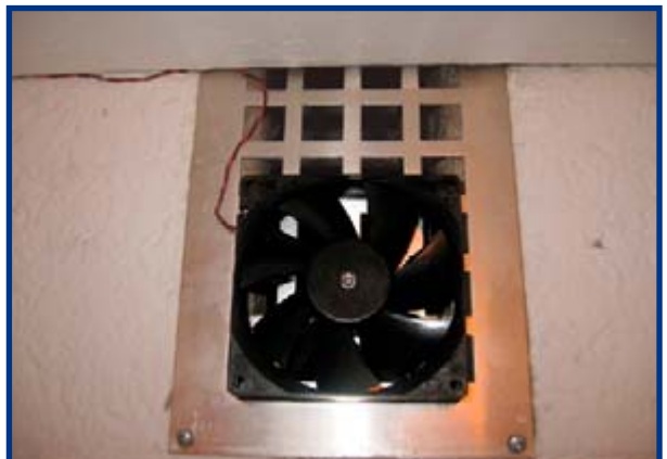
The controller could also drive other devices than the terror indicator lights. You could for example hook up a fan in parallel with the red, which helps to remove the offending smells from the toilet even quicker.
