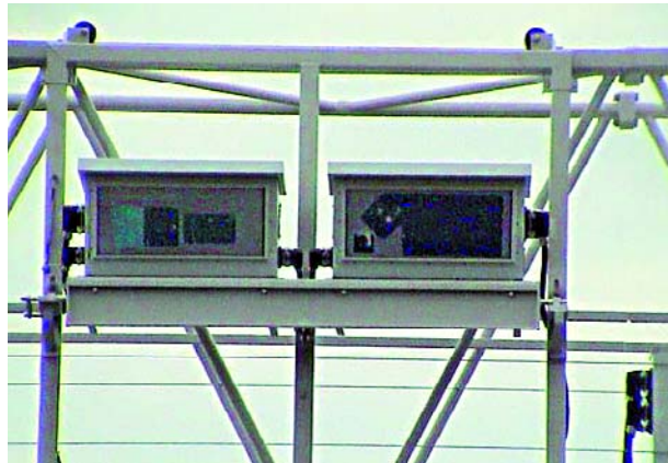
The existing motorway gantries fitted with vehicle recognition sensors for toll collection. (Picture: Toll Collect)
