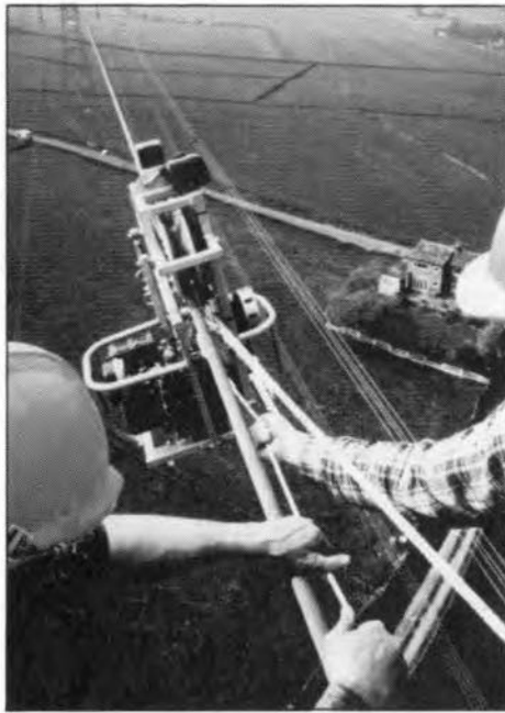
Engineers carry out the dangerous task of working on live lines, whilst installing fibre-optic cable on an earth wire of the electricity transmission network in Britain
