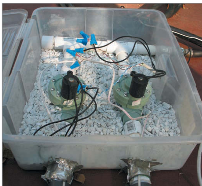
Photo 4—This valve box shows the manifold of two water valves, associated hoses, and control and sense wires.
