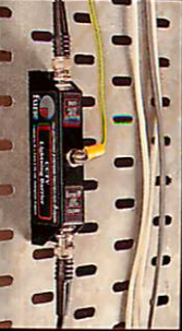
...the CCTV video cable to a security system
