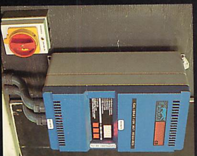
...variable speed drives
