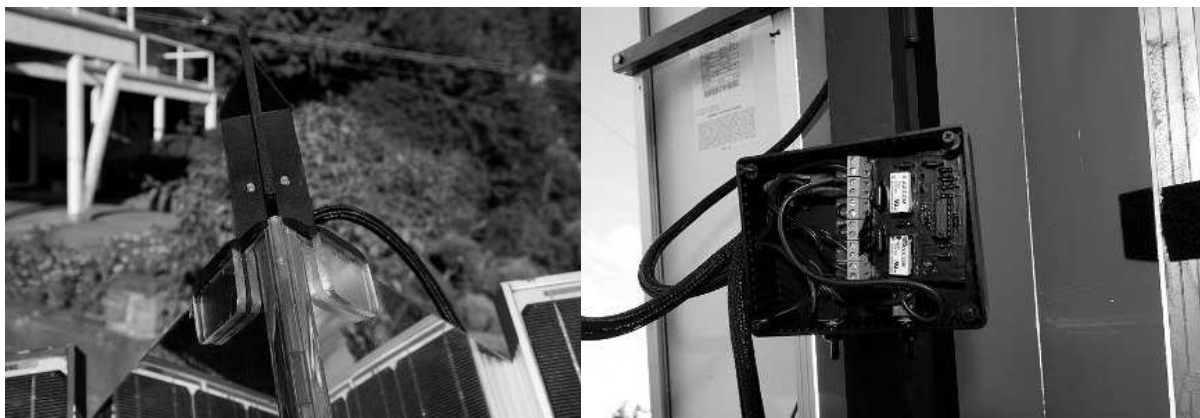
Figure 38. Here is a view of the same tracker from Figure 33. Note the the shadow block assembly. Also, note how the circuit board was ruggedized with a conformal coating and is mounted in a weather tight enclosure.
