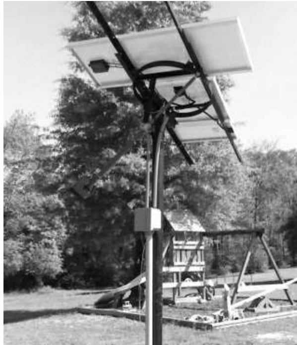
Figure 35. This Solar Tracker Project uses a DC linear actuator to move the panels. The controller is mounted inside a weatherproof electrical enclosure. The photos are courtesy of Bill F.
